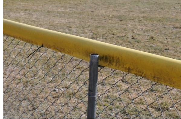
Figure 9. The outfield fence at the little league field needs repair.
